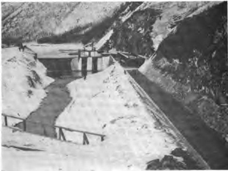
FIG. 163.—Headgates, Sluice Gates, and Sand Basins, High Line Canal, Spanish Fork Valley, Utah.
